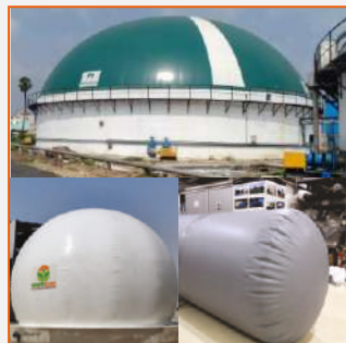
Digester & Ground Mounted Biogas Balloons/Gas Holder
