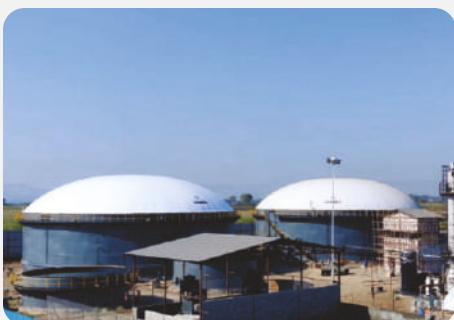
Biogas Balloons/Gas Holders
